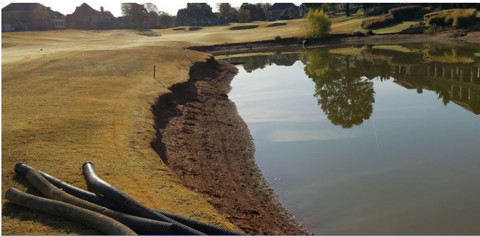
PROBLEM Substantial deterioration of pond shoreline from erosion
