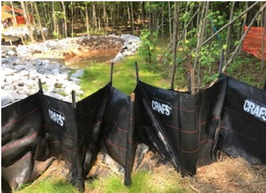
PHOTO 6 : Retained sediments are obvious within the CRAFS® “retention wedges” after one month in place and 6” rainfall accumulation. Note clarity of water in sediment pond downstream of CRAFS®. Rainfall per U.S. Weather Service. (6-2-17 Photo ID IMG-0023 LoPix)
