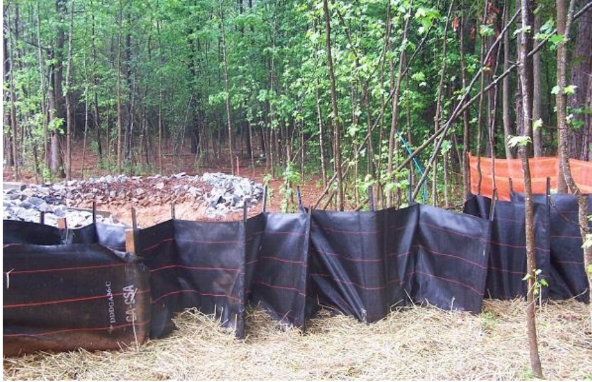
PHOTO 5 : Closer view shows CRAFS® system “in place” and stable after rainfall even Note the height of sediment deposits against adjacent silt fence fabric left of CRAFS®. Filtered seepage through CRAFS® is rapid, so sediment markings on CRAFS® filter fabric are low and hidden by the straw ground cover that’s washed against the retention wedges. (Photo ID: 100-0399 LoPix)
