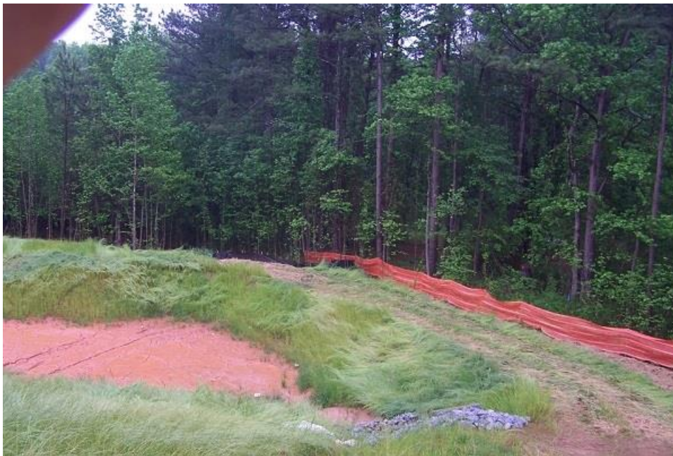
PHOTO 4 : Distant view of CRAFS® at toe of 3:1 fill slope in runoff flow path from the project's perimeter. ( Photo ID:100-0390 LoPix )
